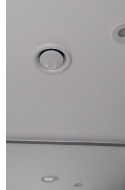
Extract grille (bathroom)
