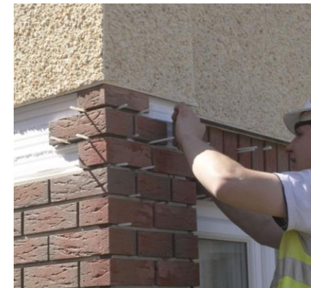
External wall insulation with brick slips in street facing facades to maintain the aesthetic
