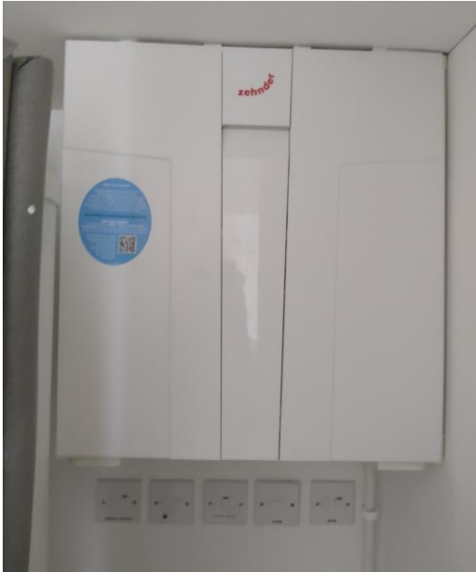
Mechanical ventilation unit
